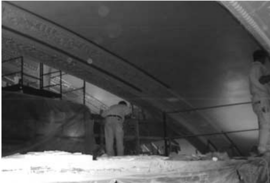
Artisan painters and renovation experts restored the interior of the Auditorium Theatre to its original grandeur public/private partnership rehab of the historic theatre.
